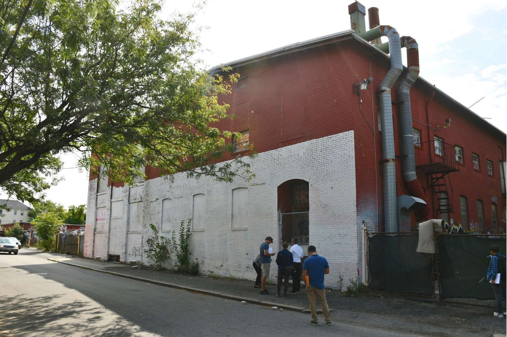
Photo #4 Building 1: Stedman & Fuller Manufacturing Company Building (right), north and west elevations, facing southeast.
