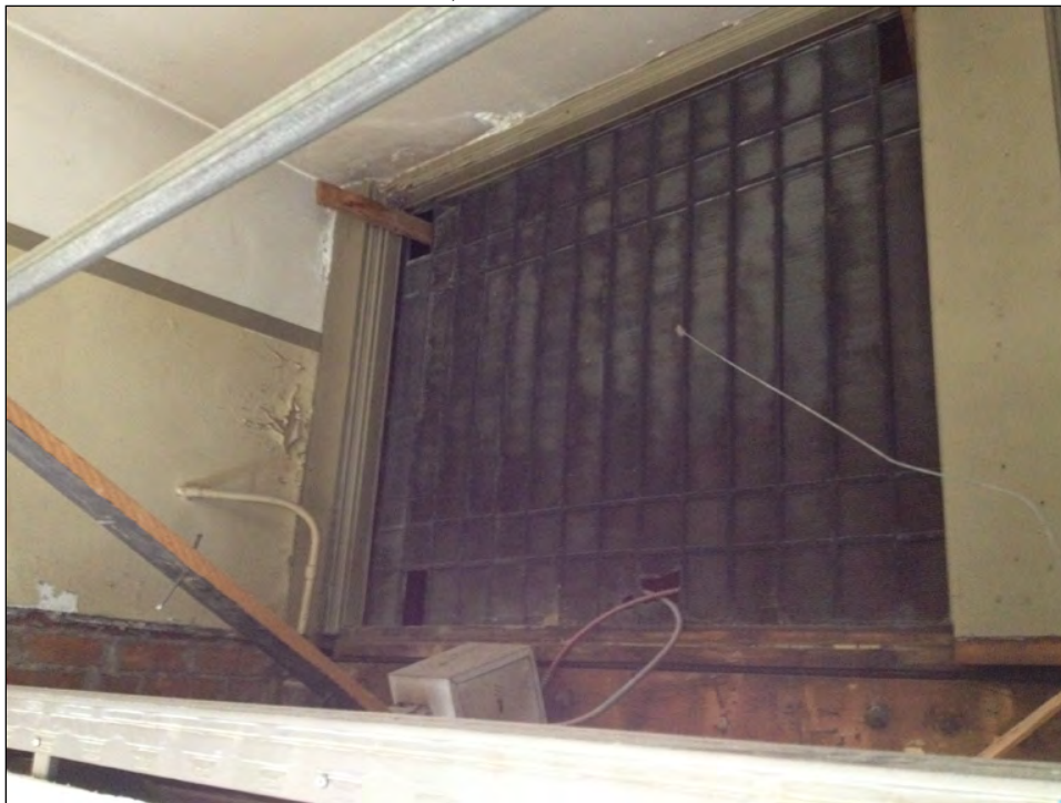
Detail of transom covered by pea stone soffit on facade and drop ceiling on interior of first floor (source: Aharonian & Associates Inc. 2017).
